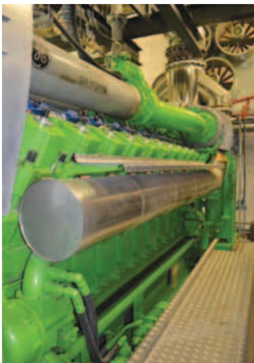
One of the four J 620s from GE installed at the Absa energy centre in Johannesburg. These 20 cylinder reciprocating gas engines have a peak generation capacity of 2,8 MW each and emit 40% less greenhouse gases than coal-based generation, making them one of the cleanest combustion based technologies available.
