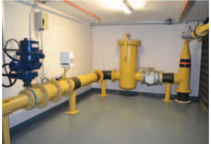
Incoming gas is at very low pressure, which makes it an extremely safe transporting mechanism. The main gas valve is held open against a spring and will shut-off automatically as soon as any sensor detects a leak.
